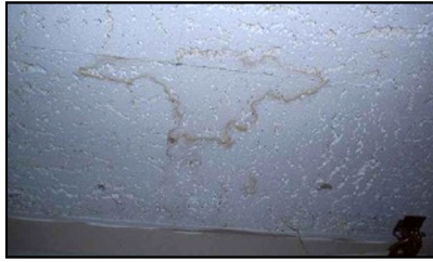
Rodent urine stain in dropped ceiling
