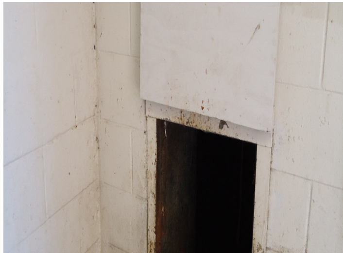
Figure 15. Poorly maintained trash chutes attract pests, providing a plentiful food supply and access to all floors of a multistory building. Photo: Dawn H. Gouge, University of Arizona
