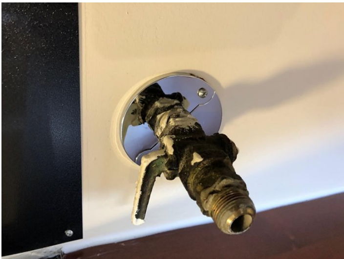
Figure 17. Deny access to wall voids by ensuring collars and escutcheon plates fit around pipes and conduits. This shows a perfectly installed escutcheon plate around a gas line installed during unit turnover. Photo: Susannah Reese, StopPests
