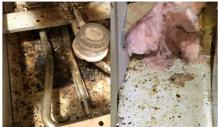
Figure 4. Droppings within the kitchen stove (left). Figure 5. Droppings in wall insulation (right). Mice leave droppings where they hide, and where they travel. Photos: Susannah Reese, StopPests
