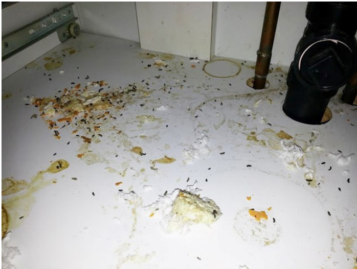
Figure 23. House mouse droppings and urine. Note the unsealed holes around the pipe penetrations. Photo: Dawn H. Gouge, University of Arizona
