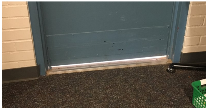
Figure 18. Light “leaks” around doorways are indicators of “open” doors for house mice. Photo: Shujuan Li, University of Arizona
