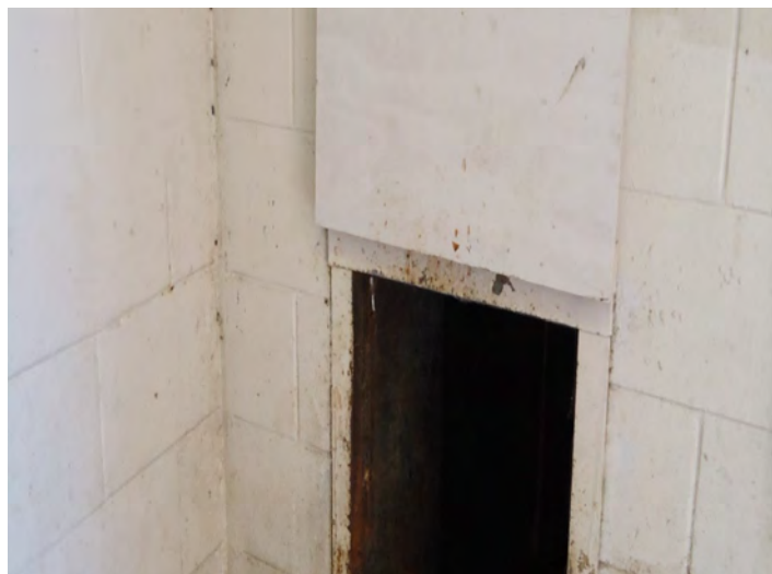
Figure 15. Poorly maintained trash chutes attract pests, providing a plentiful food supply and access to all floors of a multistory building. Photo: Dawn H. Gouge, University of Arizona
