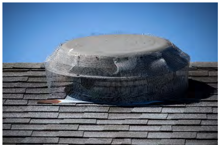
Figure 19. Exterior mesh on attic vents prevent entry for pests. Photo: Shutterstock
