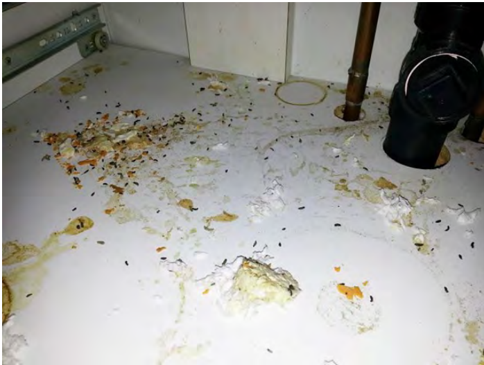
Figure 23. House mouse droppings and urine. Note the unsealed holes around the pipe penetrations. Photo: Dawn H. Gouge, University of Arizona
