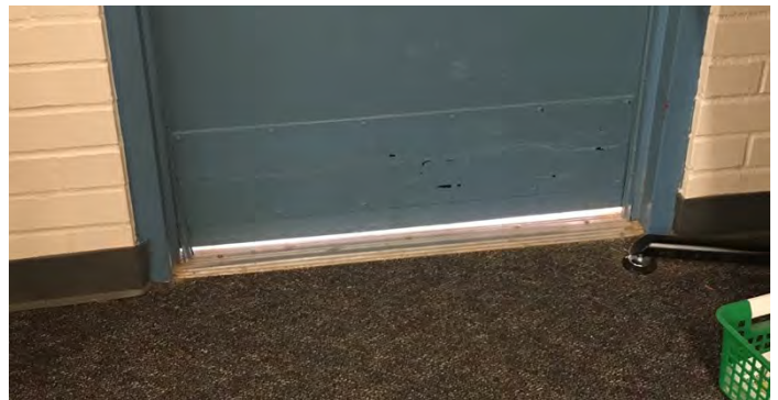
Figure 18. Light “leaks” around doorways are indicators of “open” doors for house mice. Photo: Shujuan Li, University of Arizona
