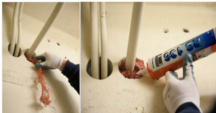
Figure 14. Seal around conduits penetrating walls. Fill gaps with rodent-proof mesh material, then seal with a siliconized acrylic latex or polyurethane sealant. Photo: Lynn Ketchum, Oregon State University
