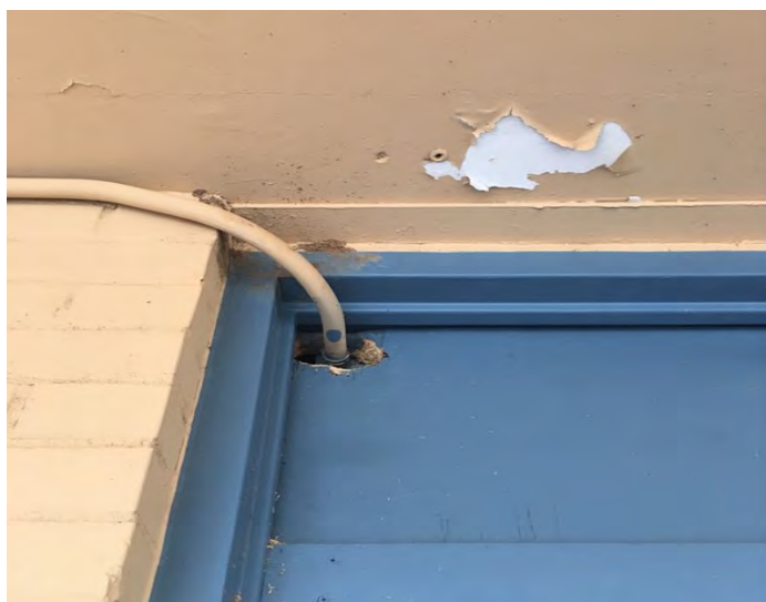
Figure 16. The gap around the wire passing through the door frame needs to be filled. Photo: Shujuan Li, University of Arizona
