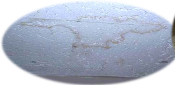
Rodent urine stain in dropped ceiling
